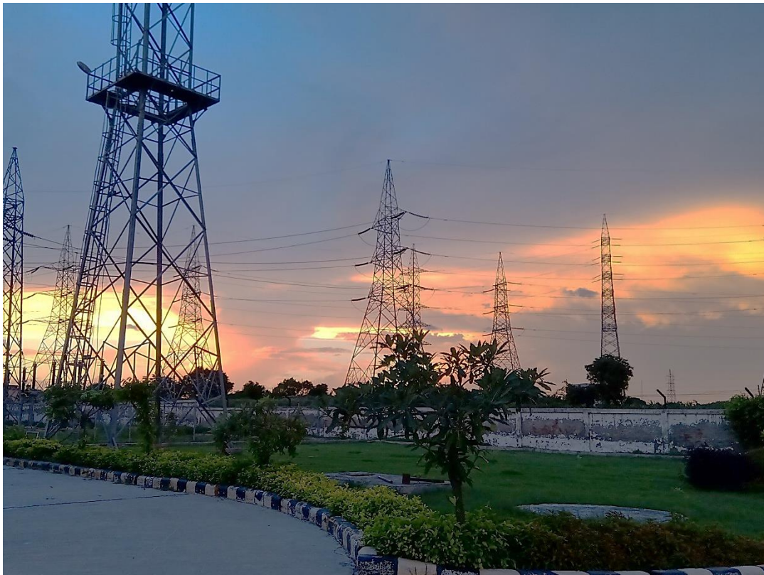
Figure 32. Lattice steel structures of overhead power lines
