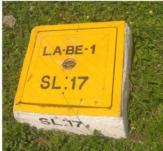
Figure 19. Earth pit with proper maintenance
