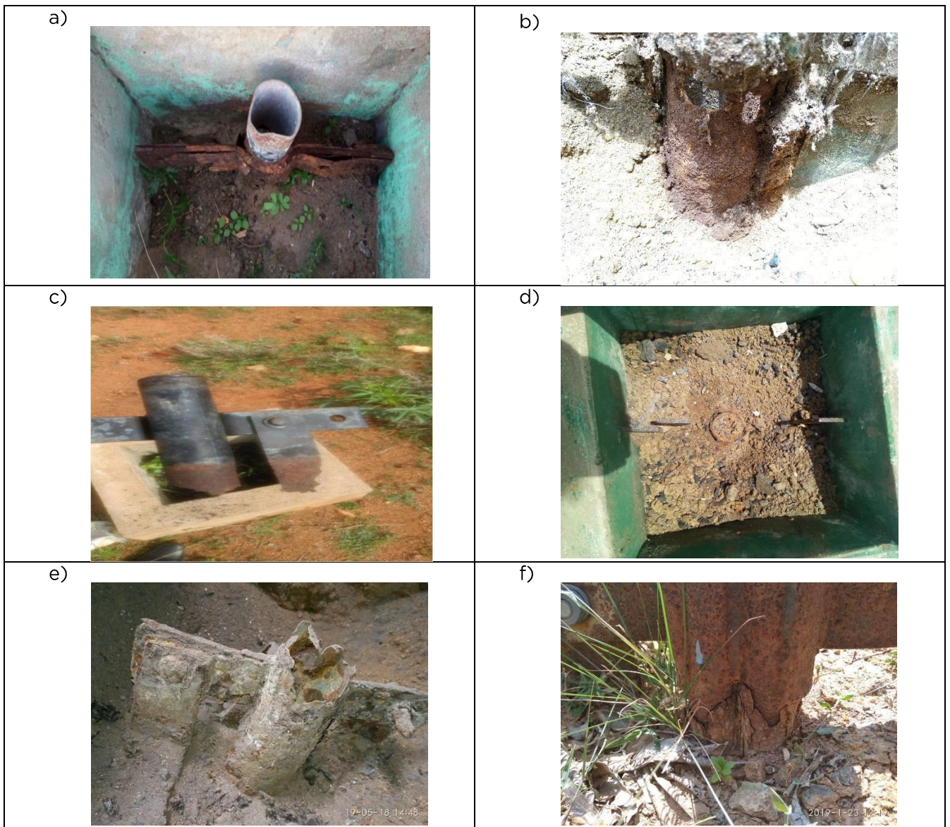
Figure 21. Corroded earth electrodes
